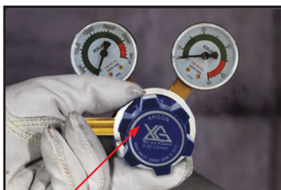
(18) Carefully open the valve of the gas cylinder, set the flow to 12-15 l/min
